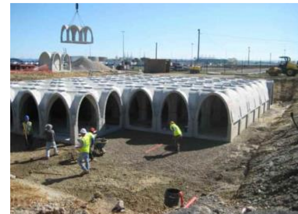
New 150,000 gallon stormwater detention vault (stormpod)
